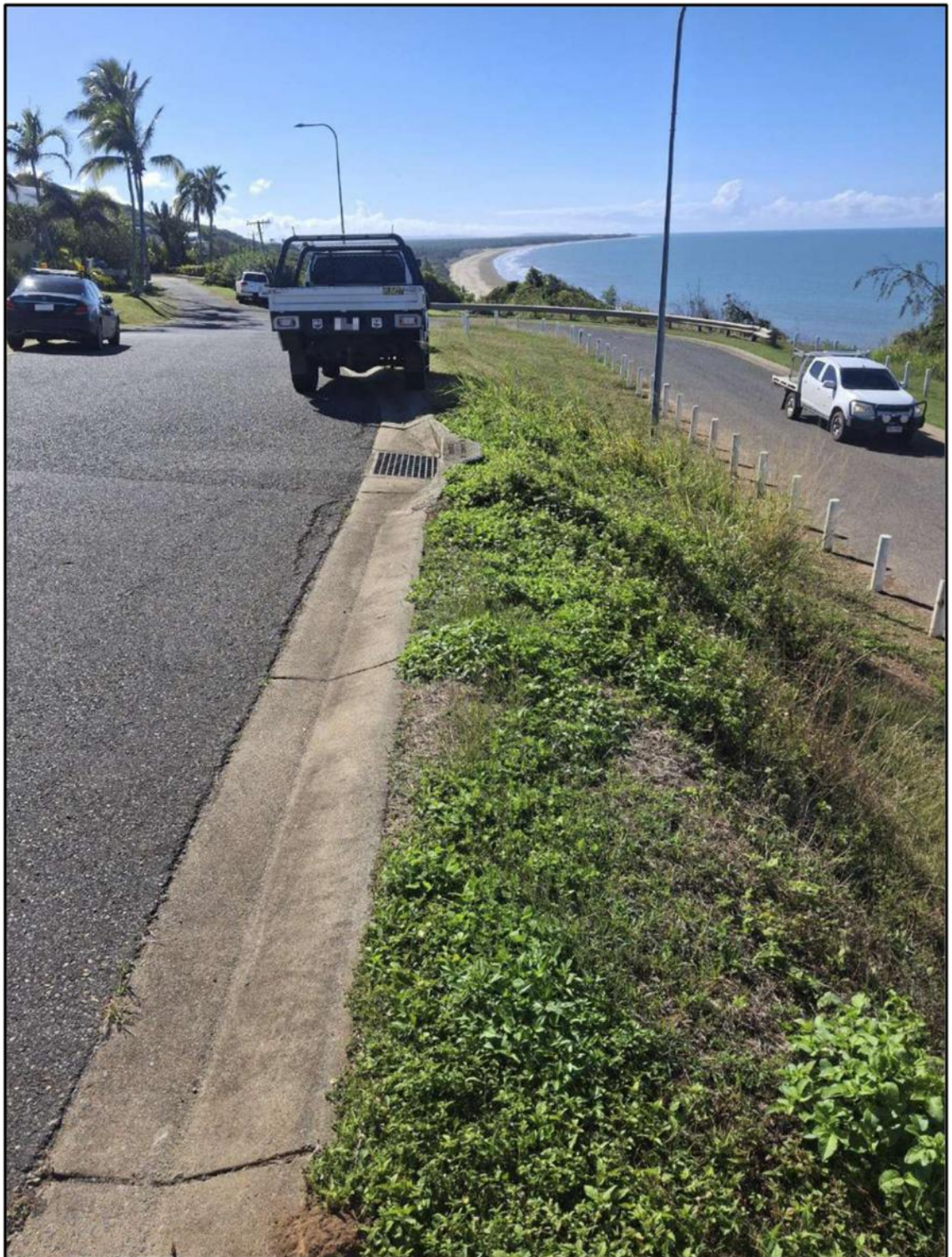
Figure 2 Vehicle Parked at Hinge of Embankment
